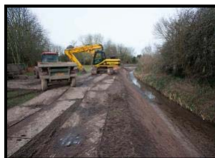
Trent Valley IDB Creating a two stage channel on the Cocker Beck
