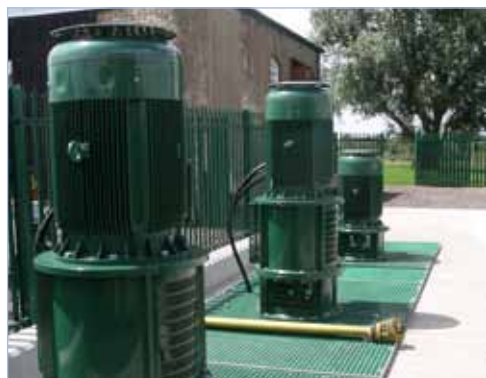
Managing Haddenham Pumping Station, Cambridgeshire
