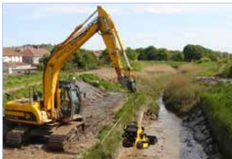
Partnership Working Caldicot & Wentlooge Levels IDB reducing flood risk in and around Newport (Source: Andrew Ross)
