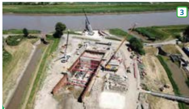
Smeeth Lode drains the area from Emneth to Terrington St Clement and is pumped via Islington Pumping Station (picture) to the Great Ouse Tidal River at Eau Brink.
