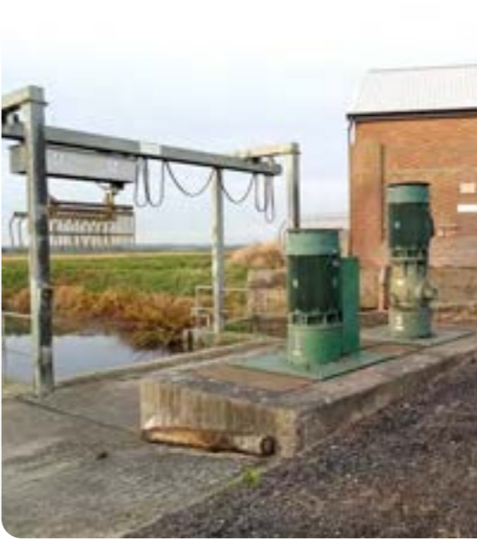
Pidley Pumping Station
