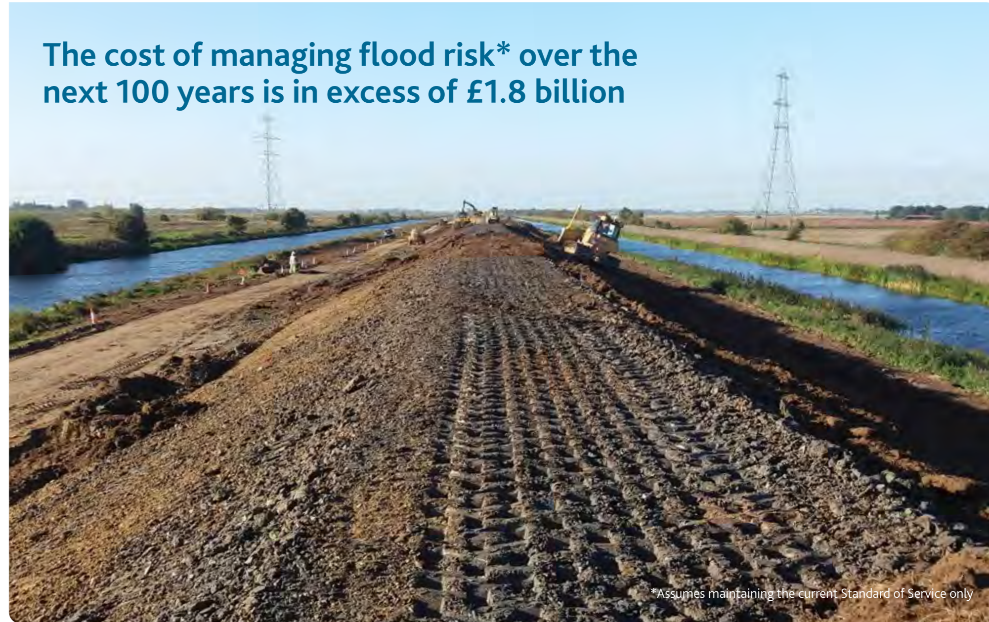
Middle Level Barrier Bank
