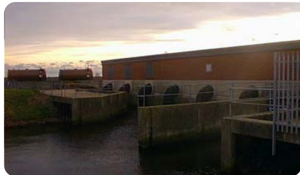
Figure 22: Bevills Leam Pumping Station, Photo: Middle Level Commissioners
