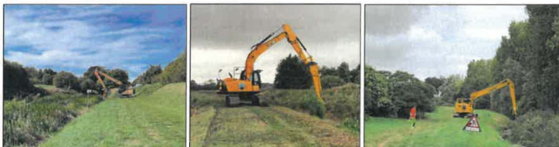
Photos 3, 4 and 5: (L) Waithe Beck (M) Oldfleet Drain (R) New Cut Drain Grimsby
