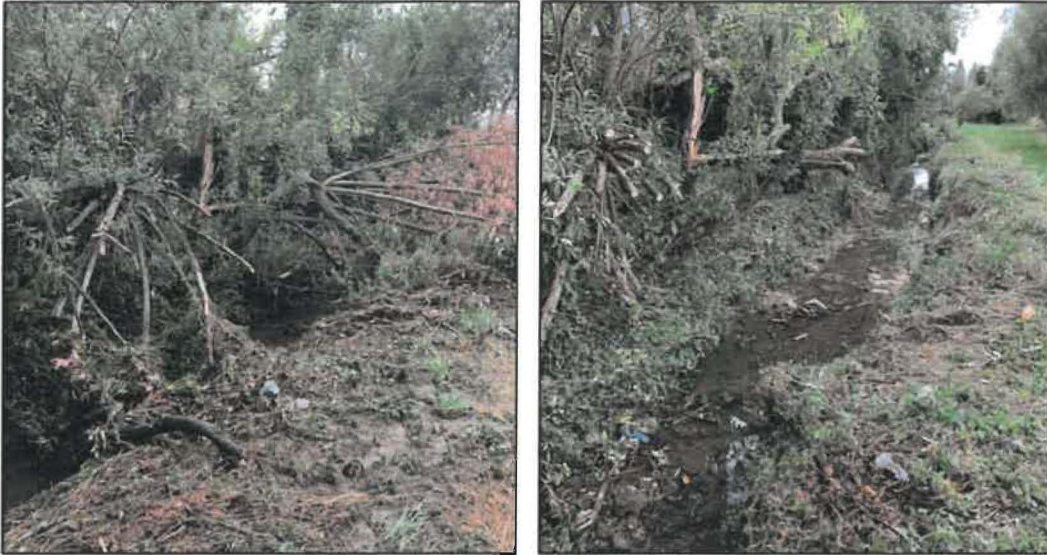
Photos 18 & 19: Removal of tree branches on Slade Brook obstructing the flow of water
