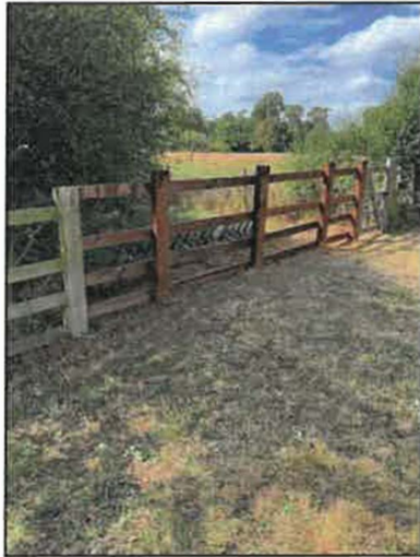
Photo 15: Fence and gate repairs on safety structures at Melbourne Flood Storage Reservoir
