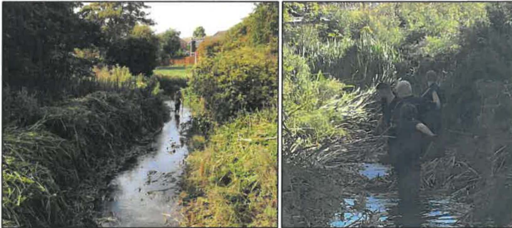
Photos 20 & 21: Vegetation clearance and incident response training on the New Cut in Grimsby
